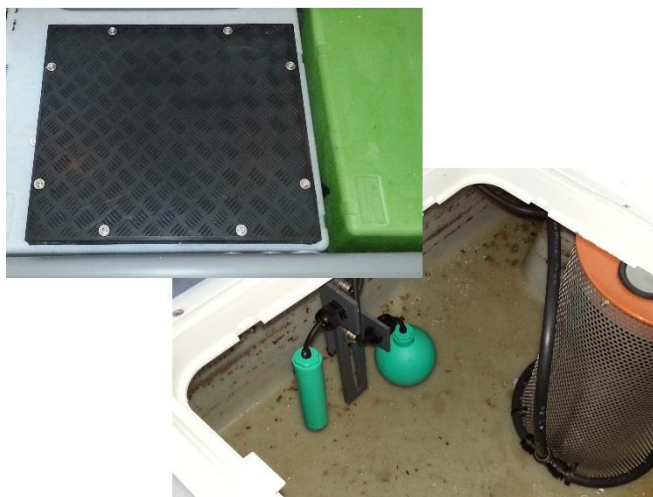
Existing waste water buffer tank turned into pre-cleaning tank and equipped with lid
