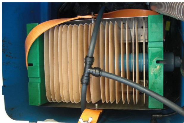
MBR tank with membrane module
