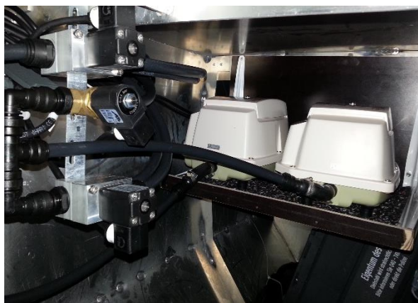
Magnetic valves and compressor in sound insulated machine room
