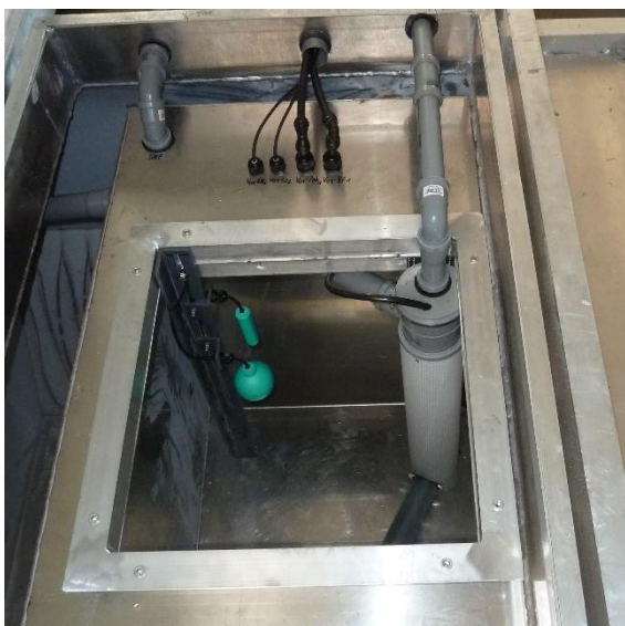
Pre-cleaning tank with pumping unit with aerated coarse matter Separator and float switch in the first floating body, open...
