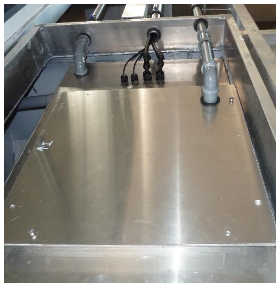
... and closed, with connection to the MBR tank in the second floating body of the floating house.
