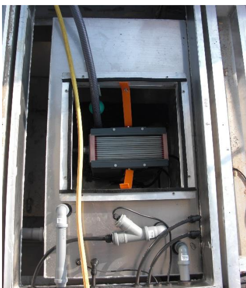
MBR tank with membrane module
