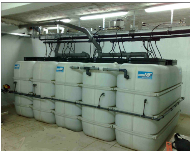
Small sewage plant with micro filtration
