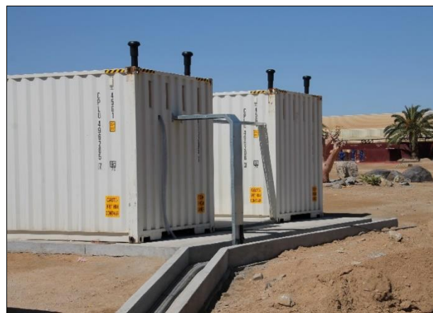
Exterior view of the waste water recycling plant, consisting of 2 x C100 conatiners
