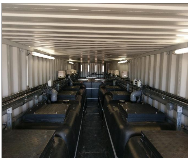
View into a container of the waste water recycling plant. You can see the membran bioreactors and the corresponding technical equipment inside the container.
