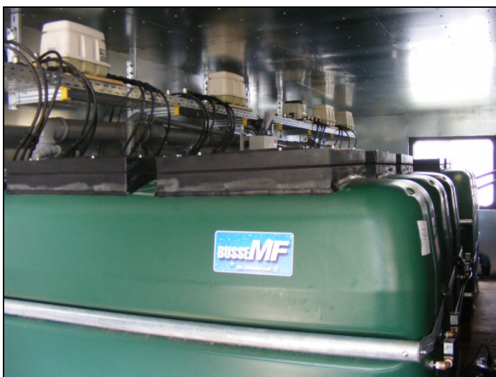
Waste water treatment system
