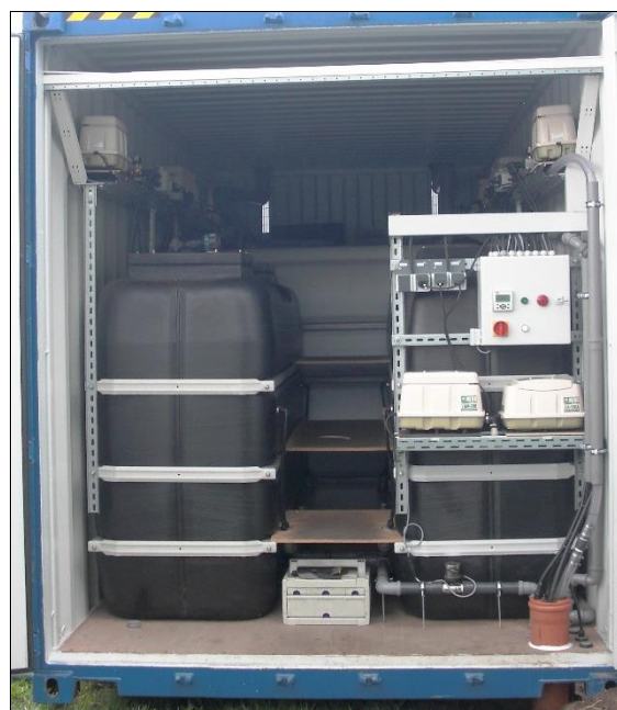
Container plant ready for operation
