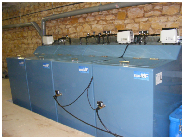
Waste water treatment system with service water storage in the school in Limeuil
