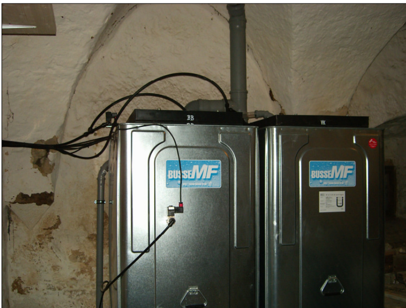
Waste water treatment system
