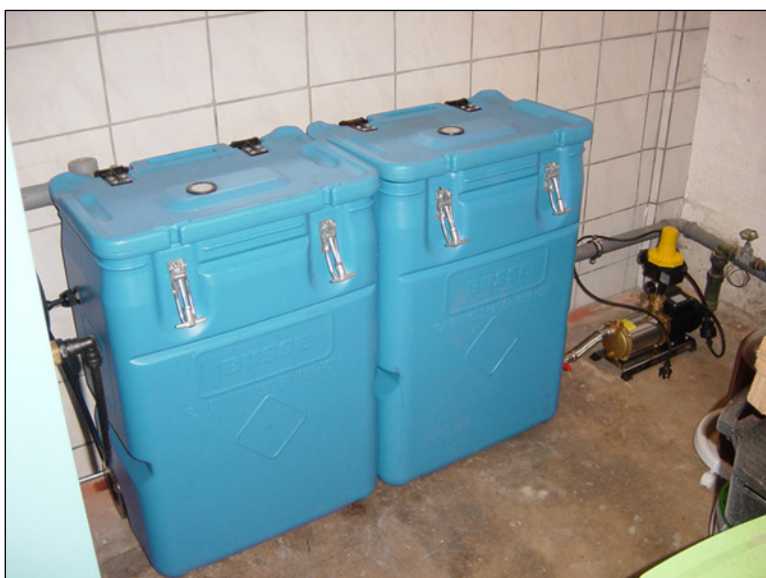
Storage for service water (300 l), home water dispenser
